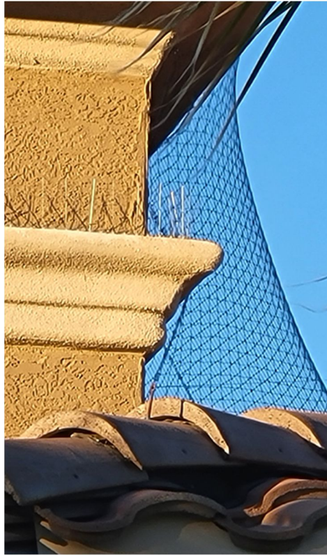
Netting in eave area between roofline changes.
